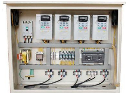
Multiple inverter systems inside layout
